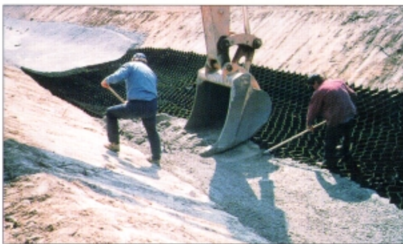
Installation of the Geoweb system was completed by a three-person crew [one equipment operator and two laborers].
