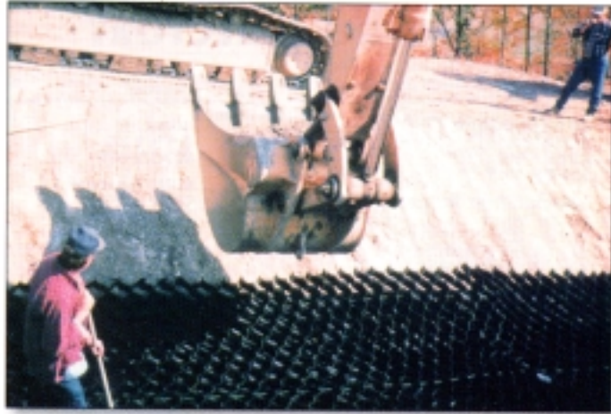
The sequence of construction was to first excavate the channel and place the nonwoven geotextile.
