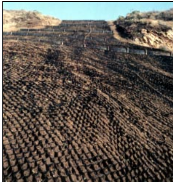
Sections of GEOWEB were stapled together for this large expanse of slope and anchored with metal stakes.
