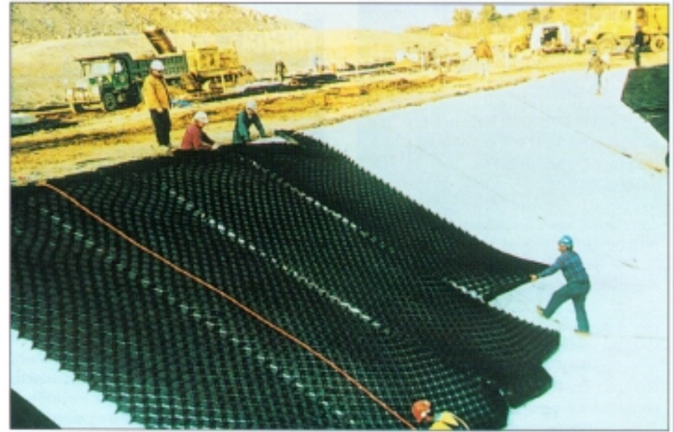
Presto's Geoweb ® sections are positioned over the GCL, expanded down the 1.5h:1v slopes and connected with a pneumatic stapler.
