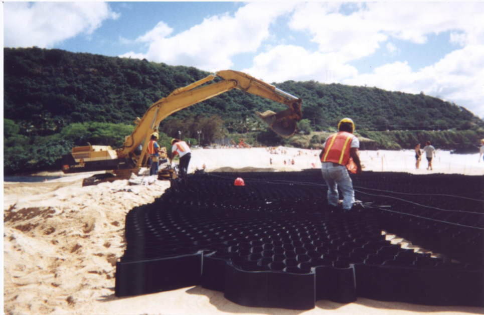
Structural Systems Inc. provided the GEOWEB material for the temporary Waimea Bay road. The contractor is Kiewit Pacific Co.
