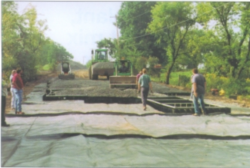
Crews lay down geotextile and Geoweb cellular confinement sections. Once the Geoweb is placed, slag aggregate is added to fill and cover the cells.
